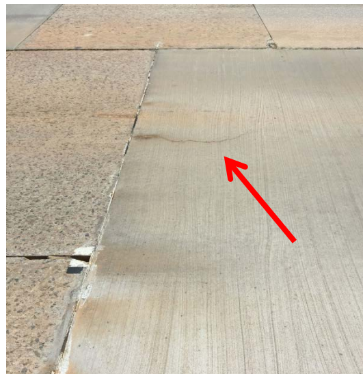
Figure 4. Control - Visible Crack Developing
