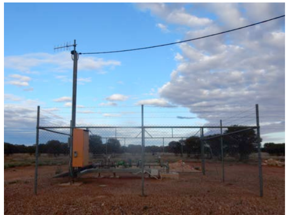
Figure 4: Local Water Supply Bore
