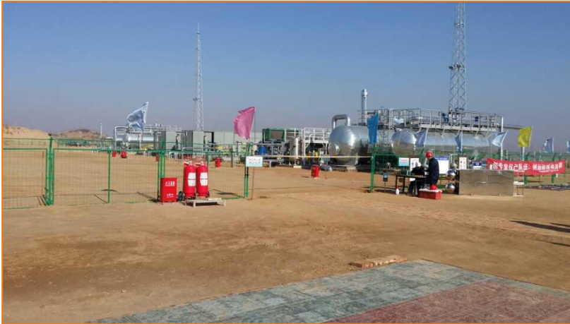
Sanjiaobei Central Gathering facilities commissioned
