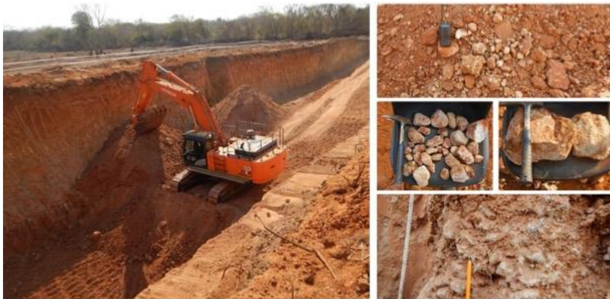
Figure 6. (i.) Excavation of Alpha Pit – depth Dug area up to 9.2m); (ii.) Gravel layer in the stock pile; (iii.) Gravel clasts of quartzite ranging from 2cm to 8cm in diameter, (iv.) Angular quartzite clasts approximately 15 cm in diameter and (v.) Gravel layer (red oxidised material with quartz clasts).
