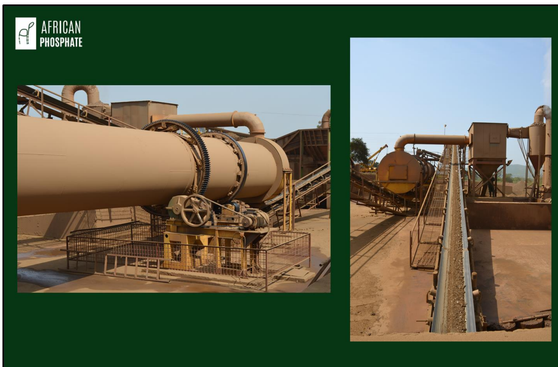
Figure 4. The Namakera Processing Plant – rotary dryer and dryer feed and discharge (Source Namakera Mining Company)
