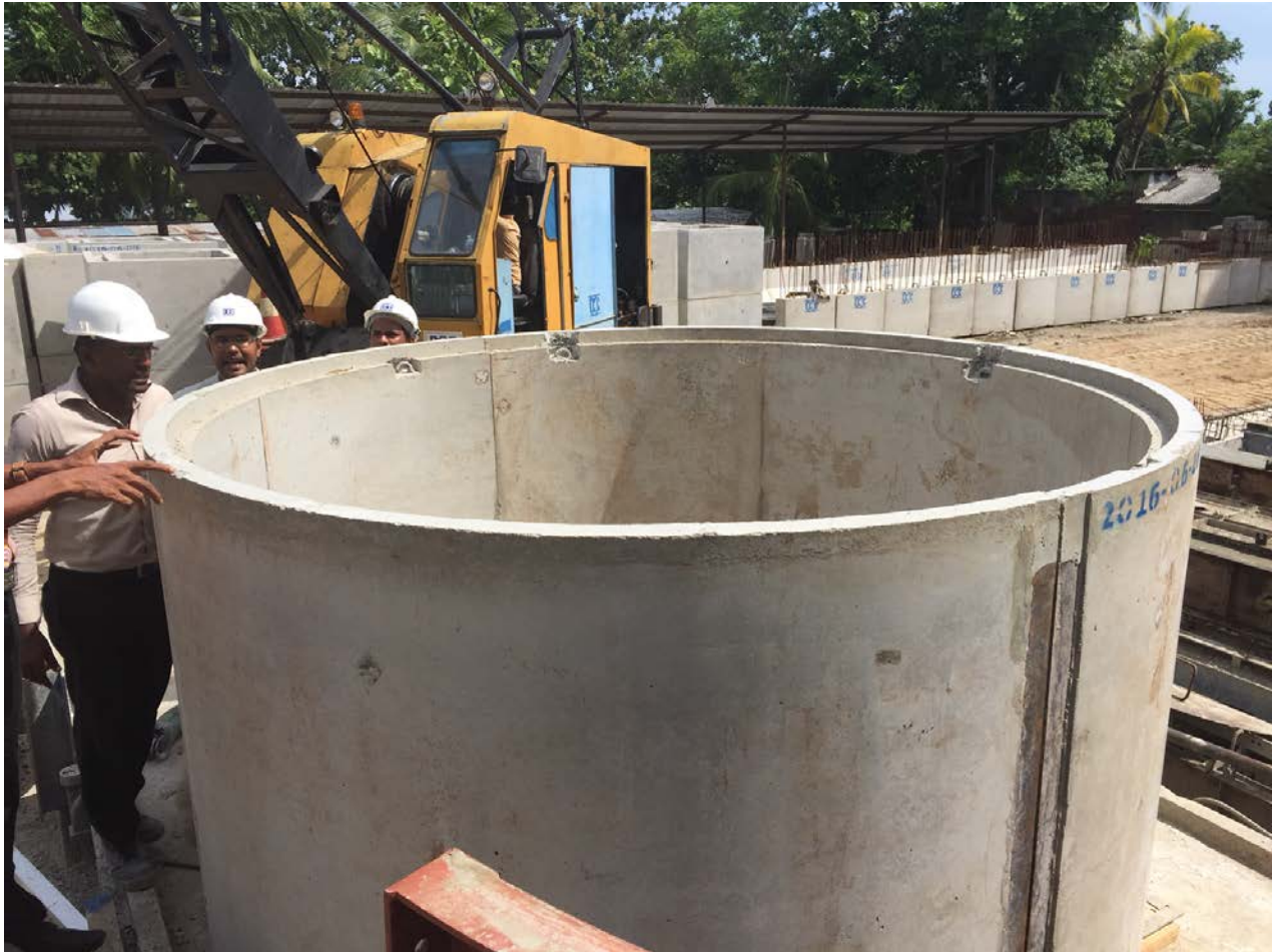
Figure 6: First trial set of 2.5m diameter shaft liners for Shaft J from FGR designed mould
