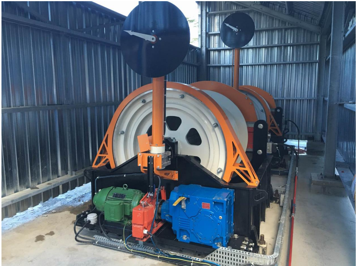
Photo 2: E15 Service Shaft Stage Winders (sinking winders)
