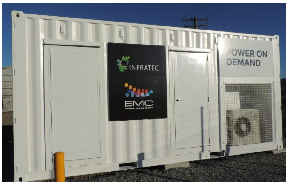
EMC's Battery Energy Storage System at the Alpine Energy's Timaru Washdyke facilities in New Zealand.
