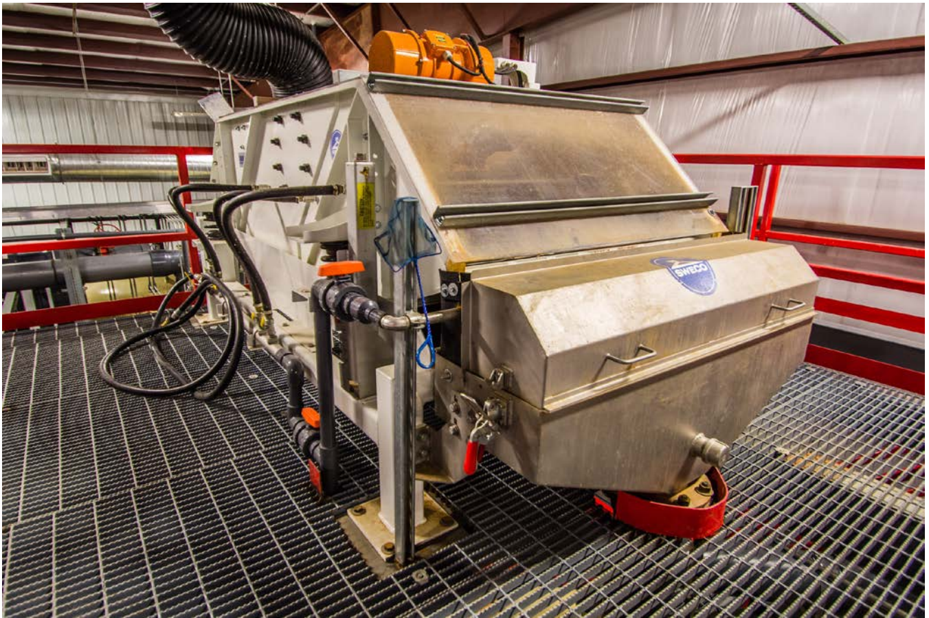
Figure 6: Resin shaker inside CPP, Lance Projects – June 2016
