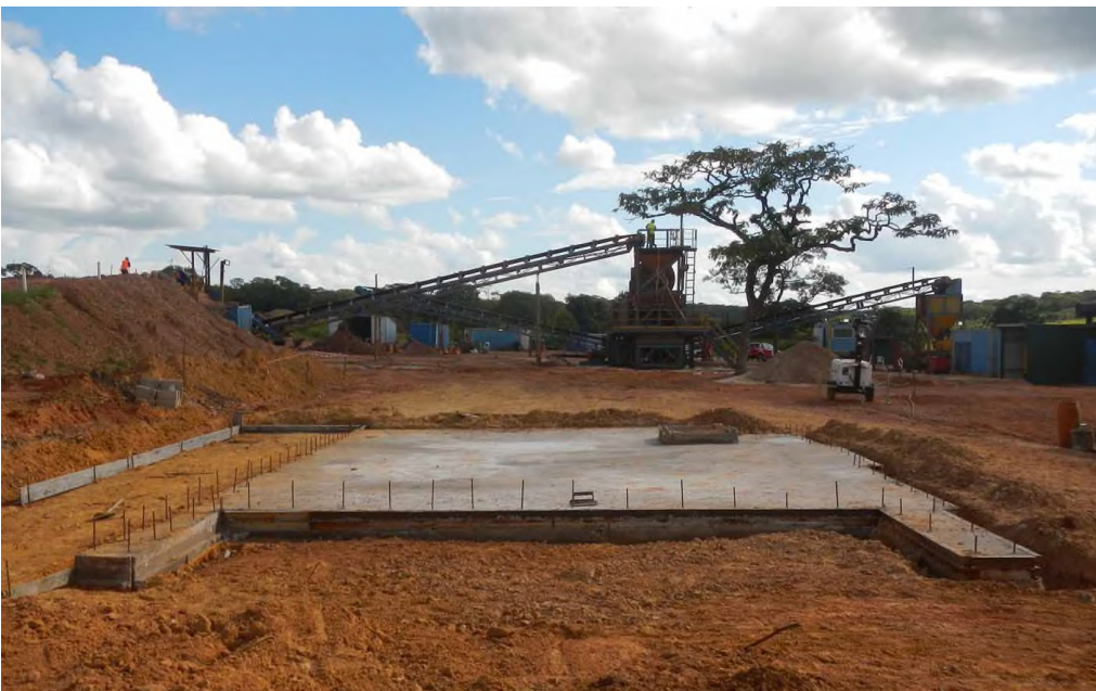
Foundations for the new wet front-end module at the 150 tonne per hour Lulo diamond processing plant
