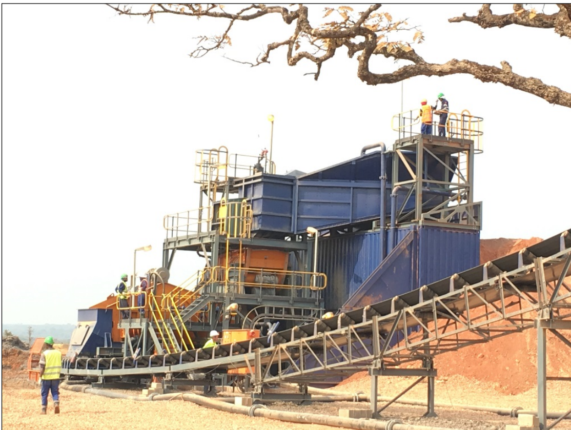
Wet front end commissioned in July 2016
