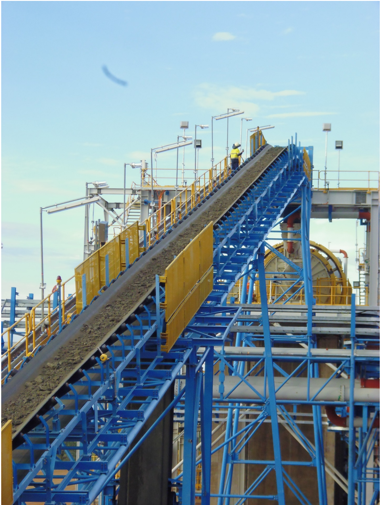
Ore feed going from the HPGR to the scrubber
