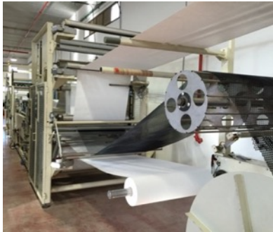
Production line in operation
