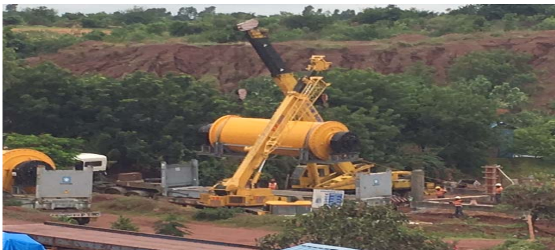
Ball Mill Unloading
