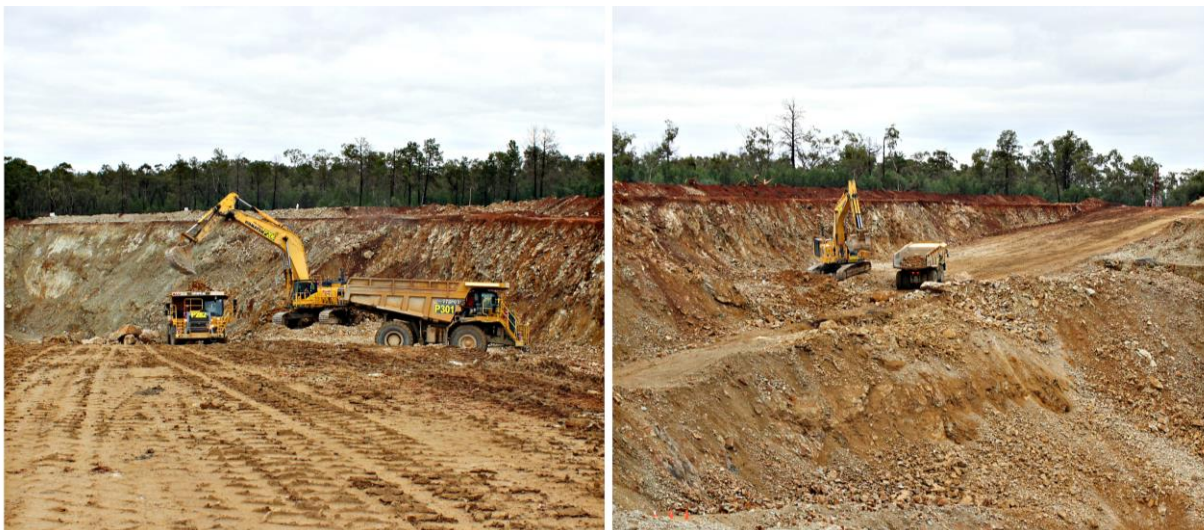
Figure 1. Pearse haul road remediation works on schedule to re-establish access for mining by mid-July.
