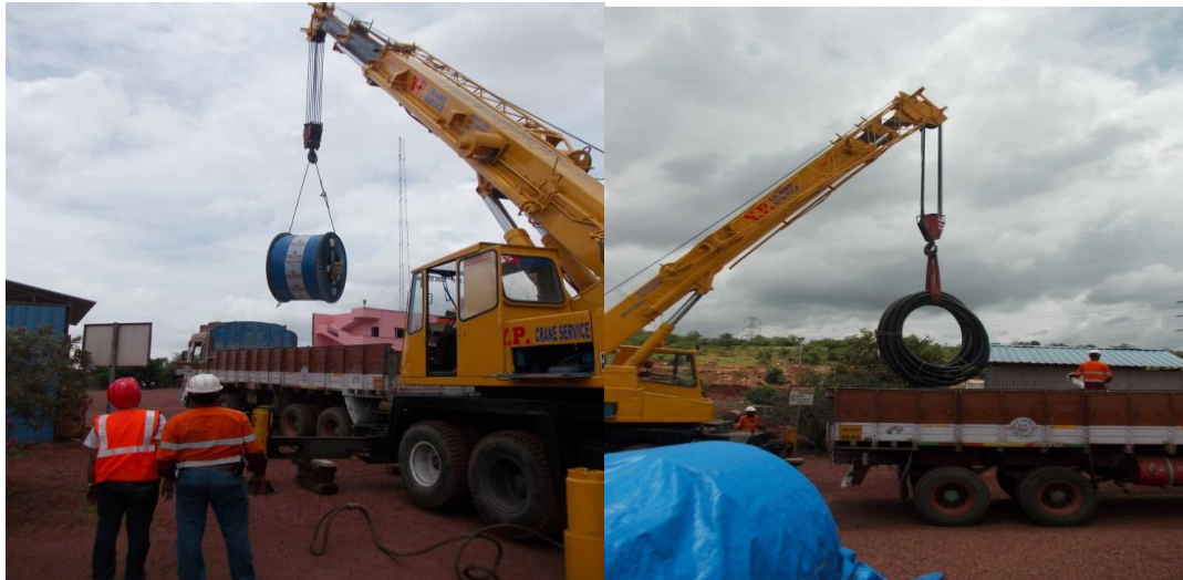
High voltage cabling arriving on site
