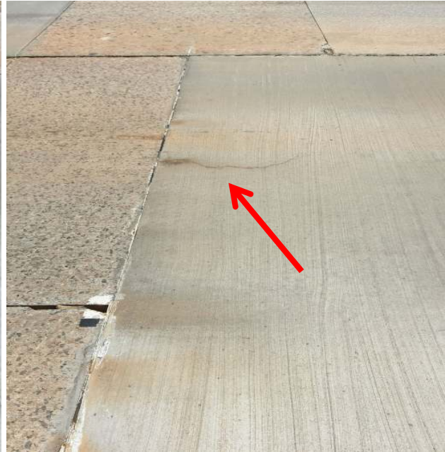
Figure 2. Control - Visible Crack Developing
