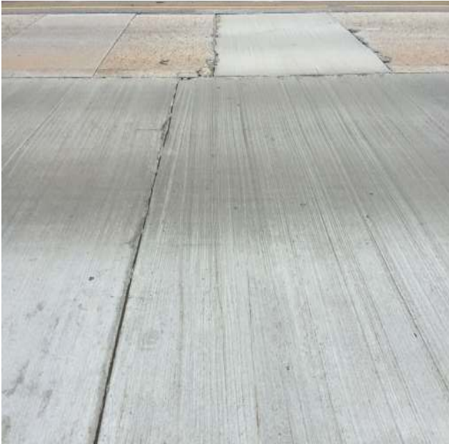
Figure 1. EdenCrete™ - No Visible Cracking
