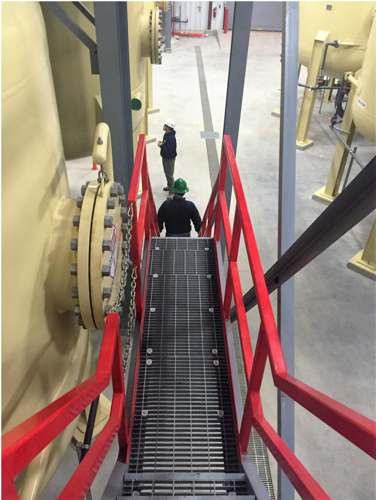
Figure 5: Ion Exchange Columns inside CPP, Lance Projects – April 2016
