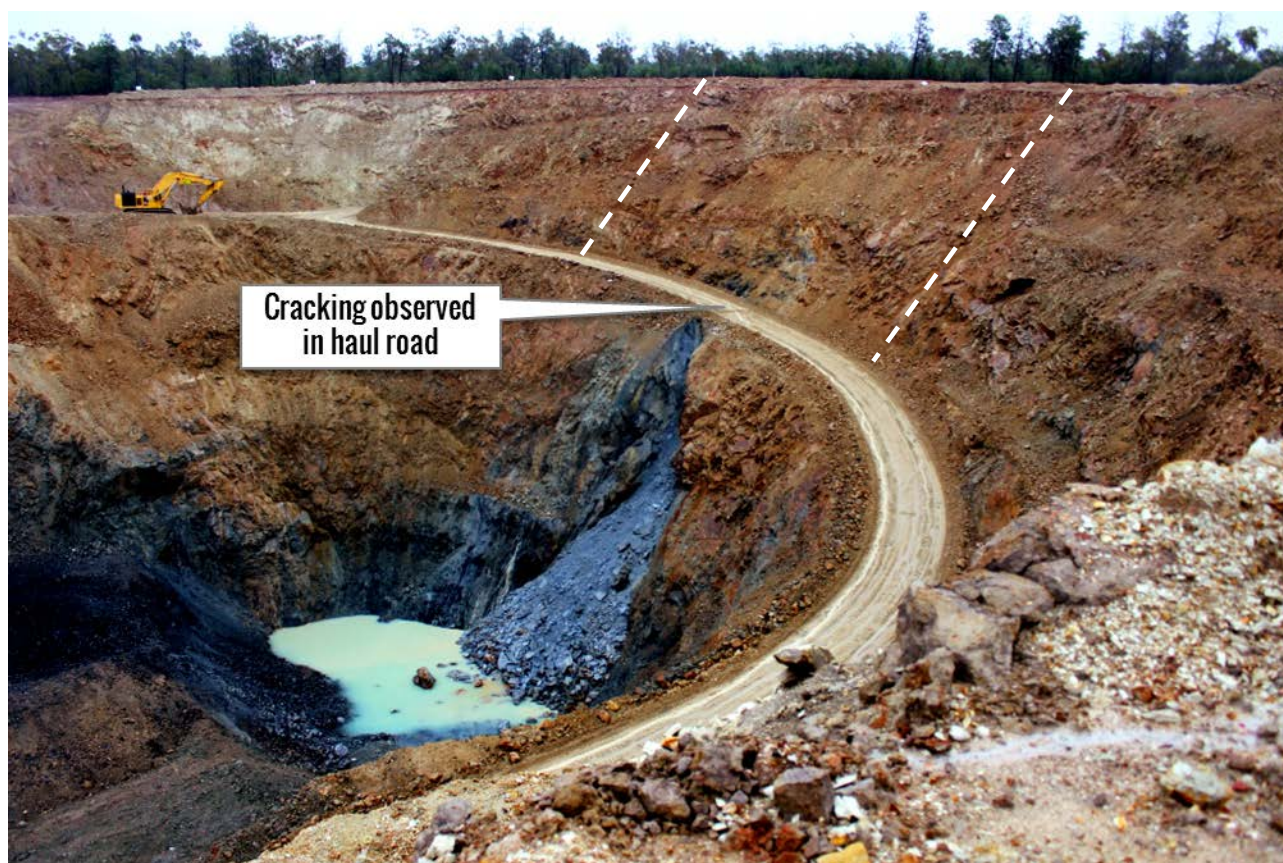
Figure 1. The Pearse Open Pit looking northwest illustrating the slip and associated cracking in the haul road. This structure represents the termination of the main shear zone in the northern wall of the pit with remedial works to relocate the haul road to the north of its existing position. The area between the lines is where some 45 kbcm of material will have to be moved to enable redirection of the haul road.
