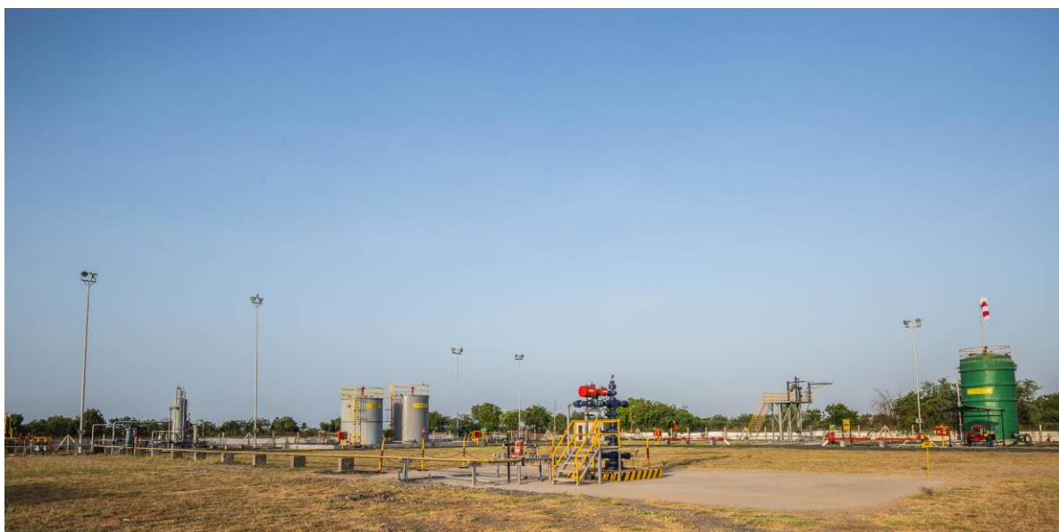
Figure 4: Cambay-73 Production Facility
