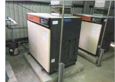
Compressed air plant
