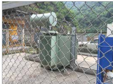
Transformer at lower portal substation S7
