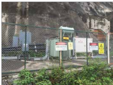
Transformer at upper portal substation S04
