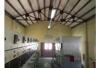
35kV / 6.3kV sub station
