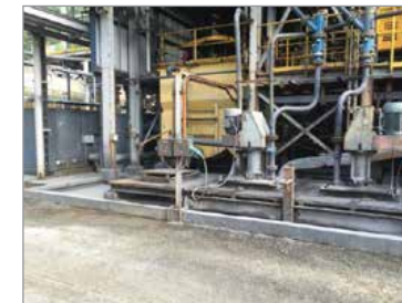
Flotation circuit tails pumps
