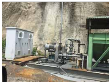
Tailings booster pump station
