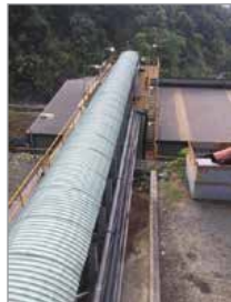
Conveyor to concentrate shed
