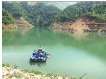
TSF pump pontoon
