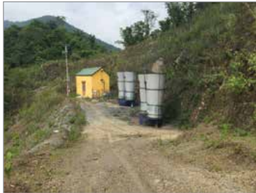
Surface vent fans and substation S5B
