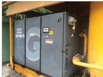
Underground air compressor #5
