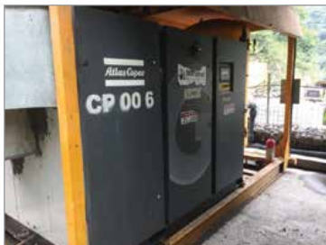
Underground air compressor #6
