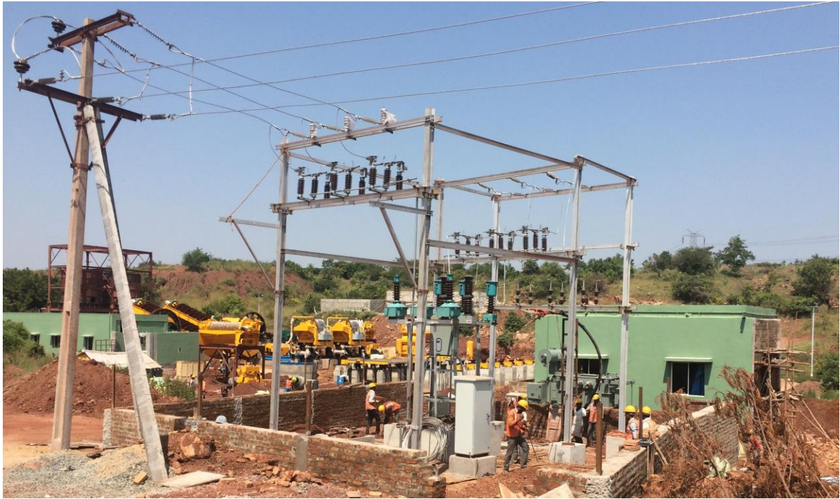
Switchyard to Main Transformer
