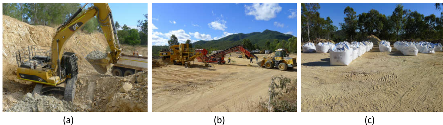
Figure 1 – Norton Bulk Sampling - (a) Bulk Sampling Frampton Shear (b) Setting up Crushing and Screening Equipment (c) Bagged Bulk Samples ready to be loaded
