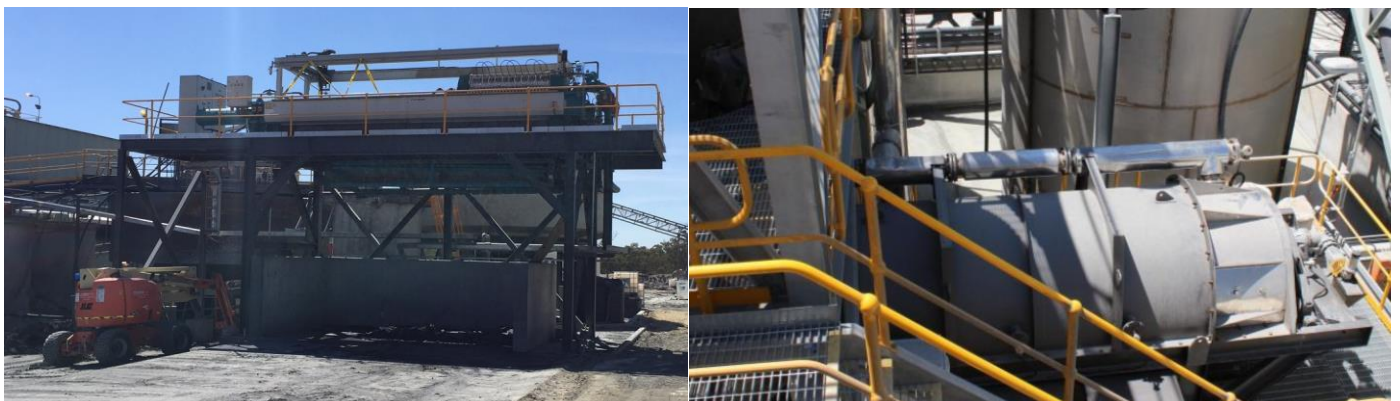
Photograph 3. New second concentrate filter and CIL carbon regeneration kiln
