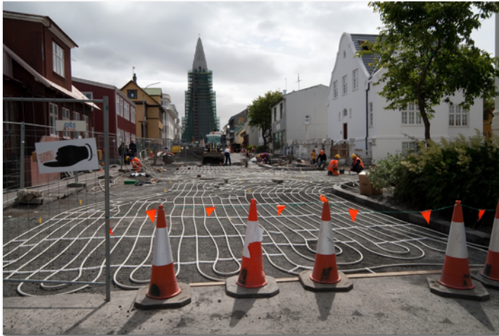
Municipal level road heating installation
