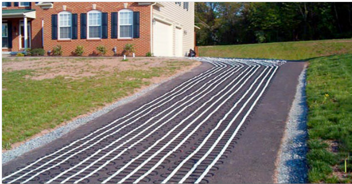
Domestic driveway heating installation
