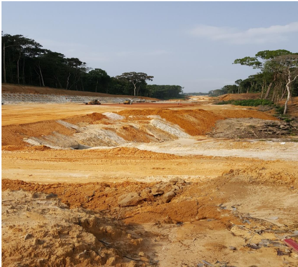
Figure 1: Construction underway of the road and rail corridor immediately east of the Kribi Deep Sea Port
