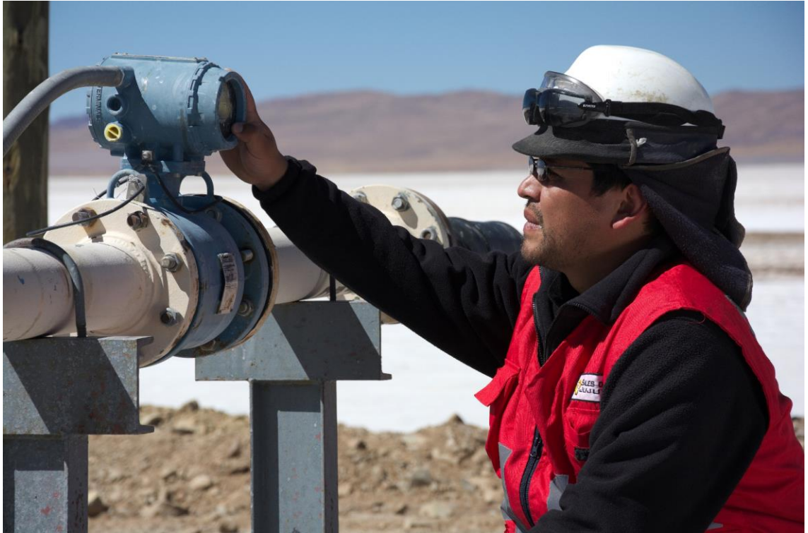
Borefield – flow rate monitoring
