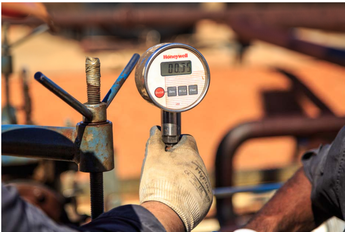
Figure 3: Mereenie; Preparation for pressure testing to recommission plant.
