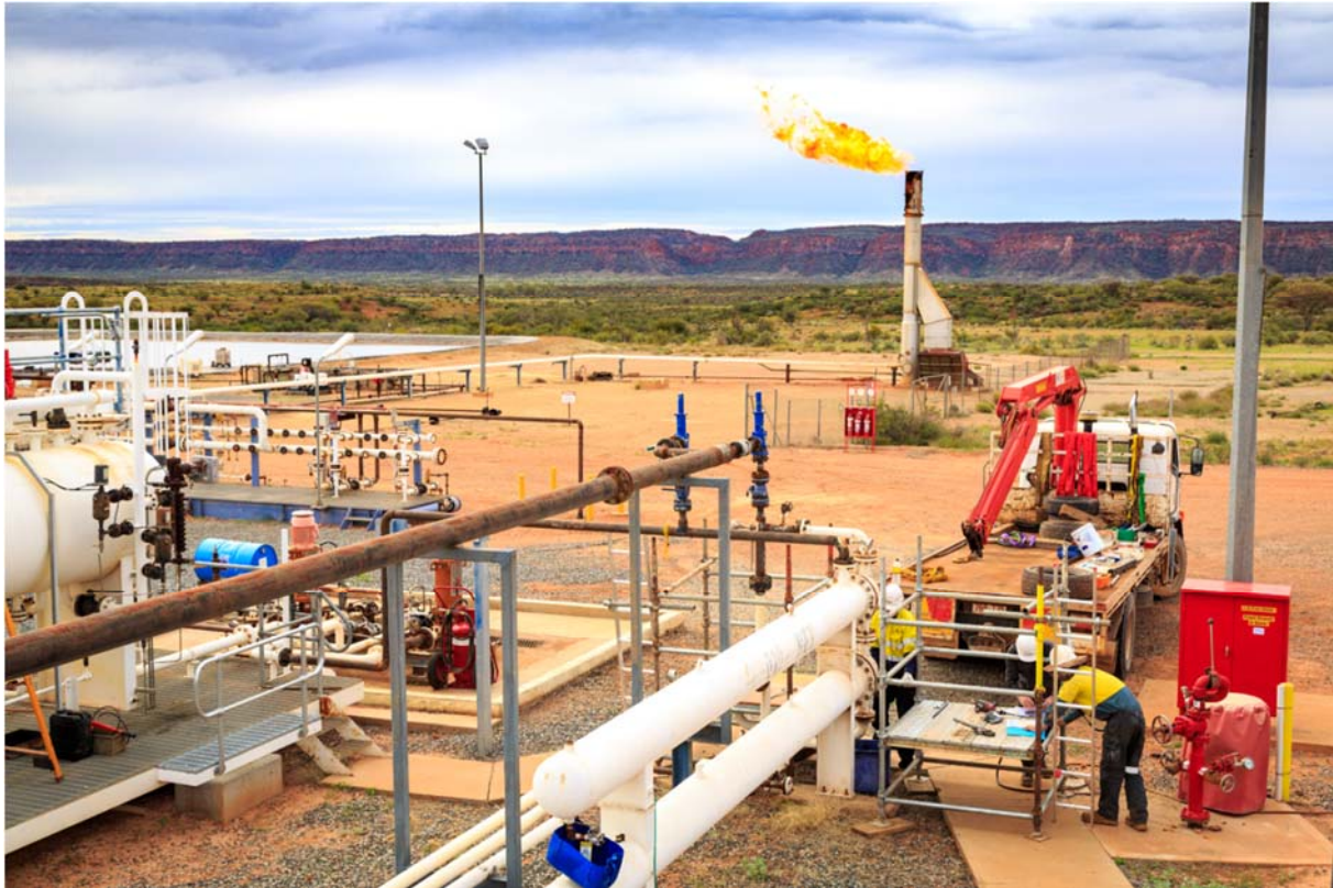
Figure 2: Eastern Satellite Station flaring while performing routine maintenance.
