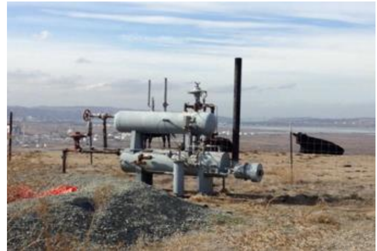
Production Facilities for early Cash Flow
