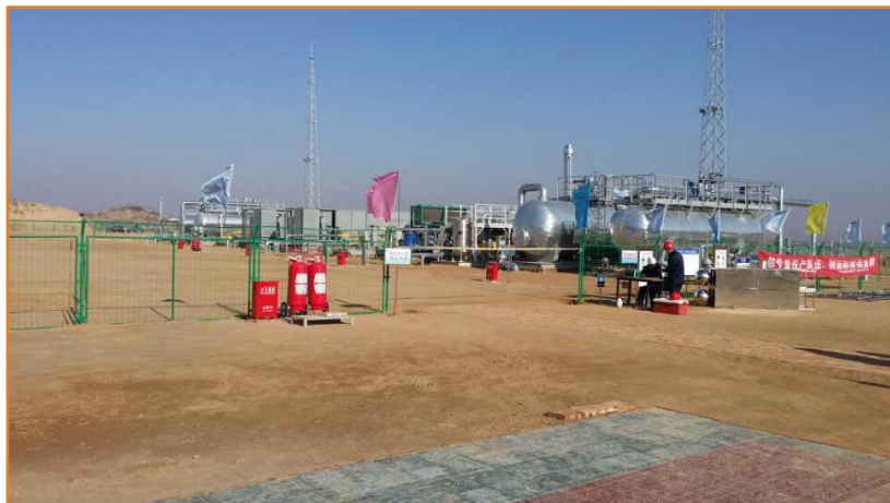
Sanjiaobei Central Gathering facilities commissioned
