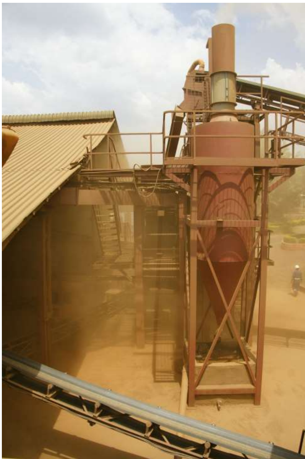
Photo 12: View of Plant Showing Feed Hopper Located on ML4651
