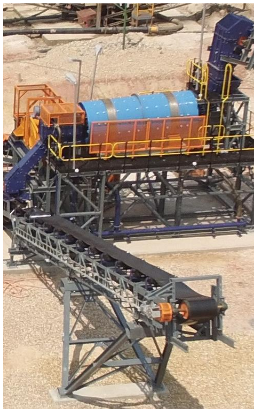
XRT Scrubber module at the 150tph diamond plant
