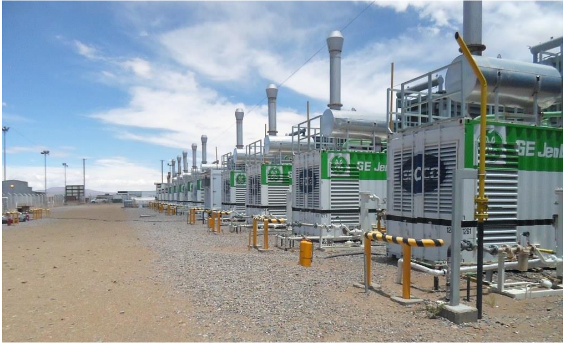
Gas generator power station at Olaroz
