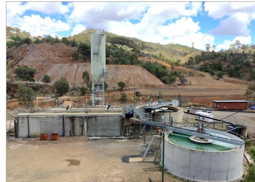
Mount Morgan water Treatment Plant
