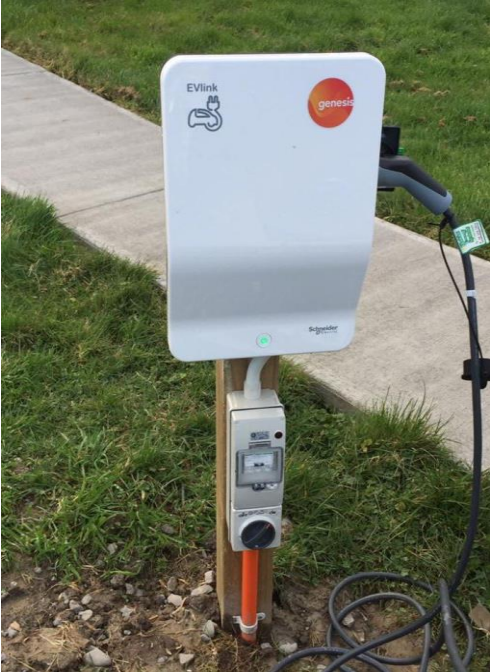
New EV charger installed at the Local Energy Project
