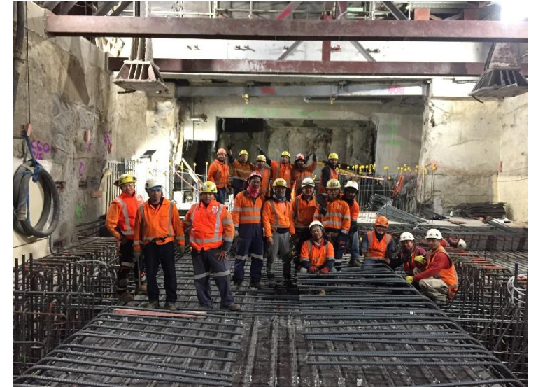
Installation of epoxy coated reinforcing in the City Rail Link project in Auckland
