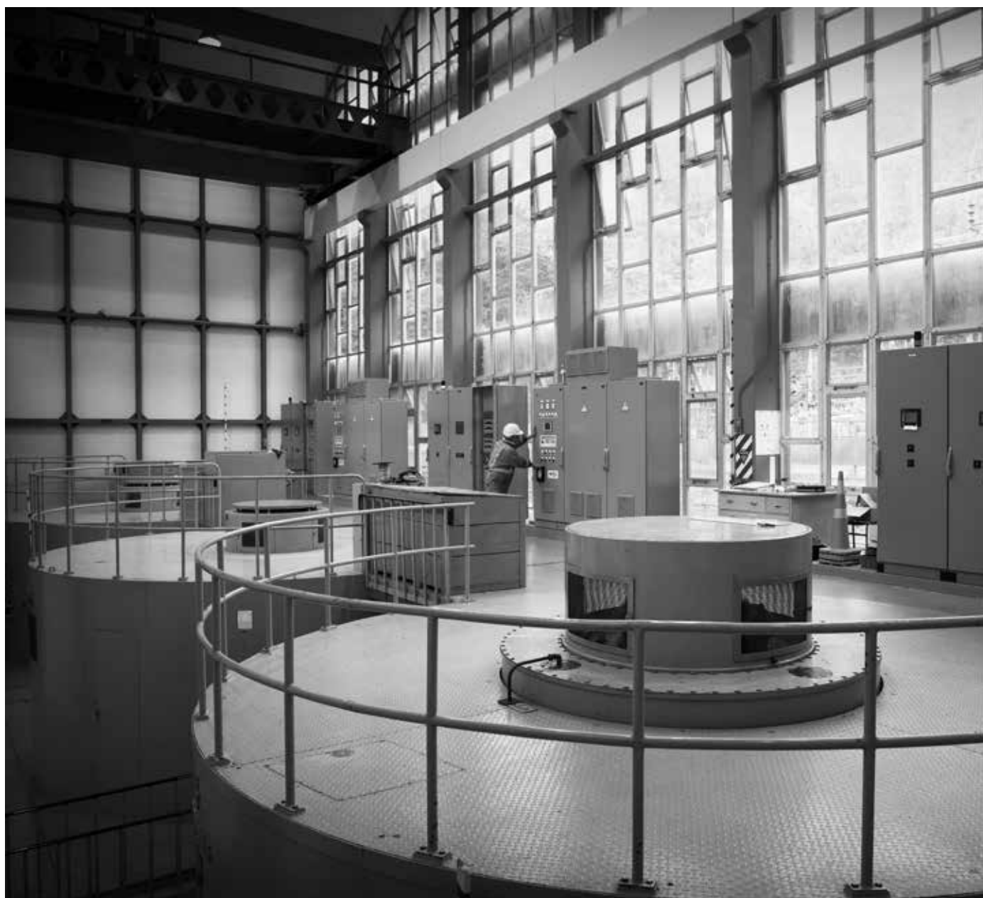
Waipori Power Station.
