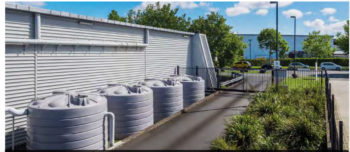
NZ Post, Highbrook Business Park: rainwater harvesting
