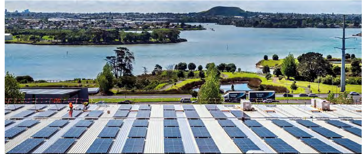
OfficeMax, Highbrook Business Park: 880-panel solar array
