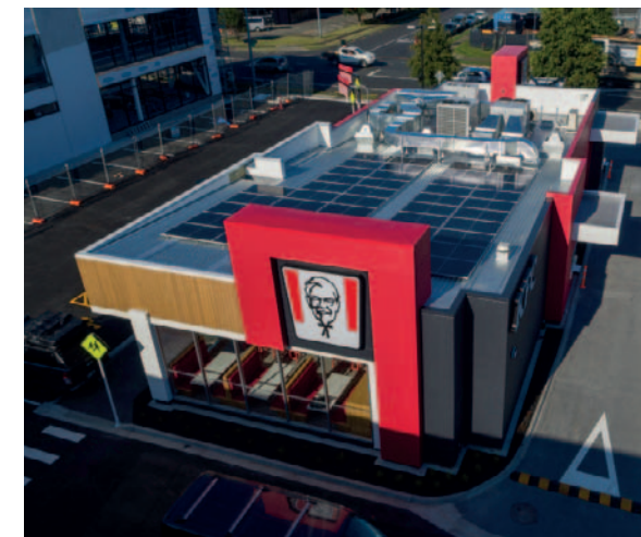
TAKANINI RESTAURANT SOLAR PANELS
