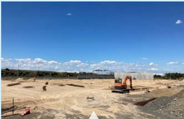
The Hamilton building site in February 2022 showing concrete tilt slab going up
