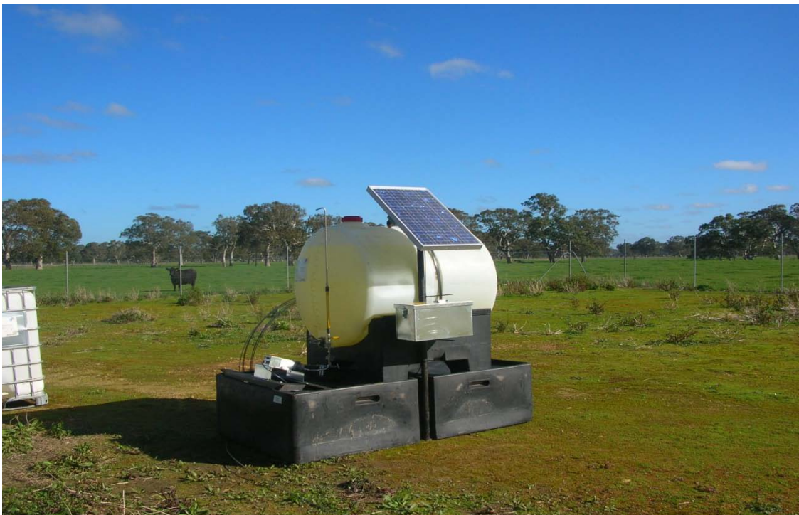
Figure 2: The solution injection tank and solar powered injection system at Haselgrove 1 Production Well Site
