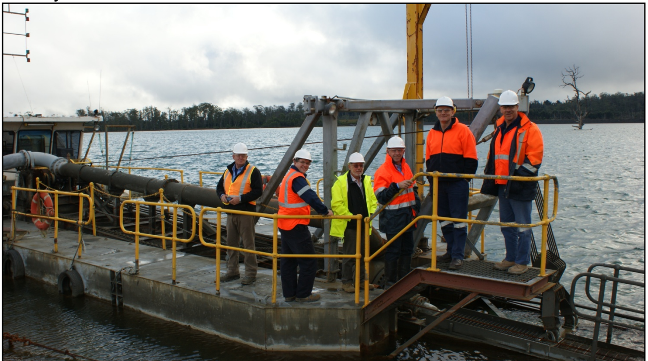
Figure 1: "The BSM Crew" aboard the cutter suction dredge on care & maintenance on the Hellyer TSF.
