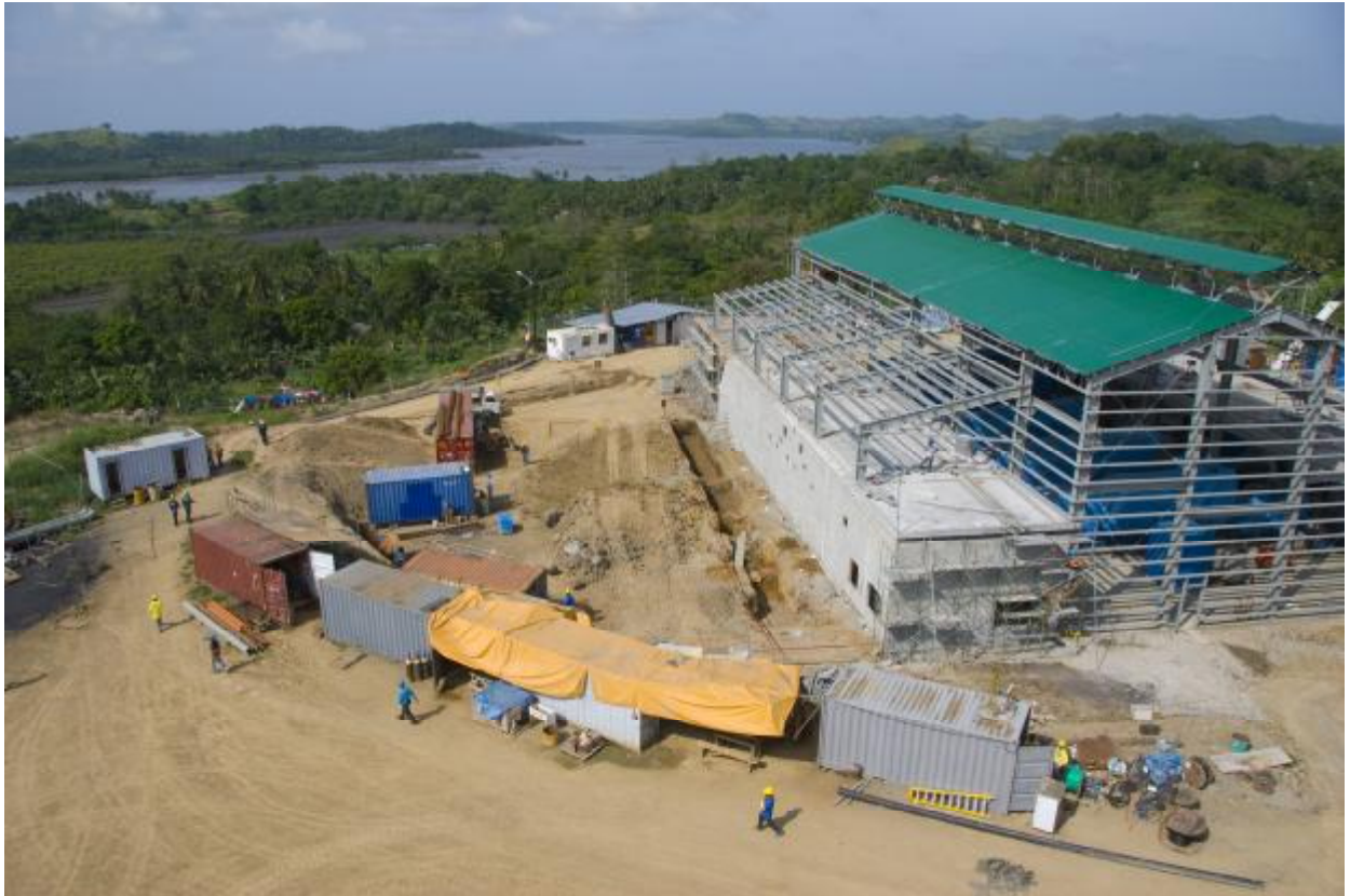
Masbate Power Plant as at 16 January 2009
