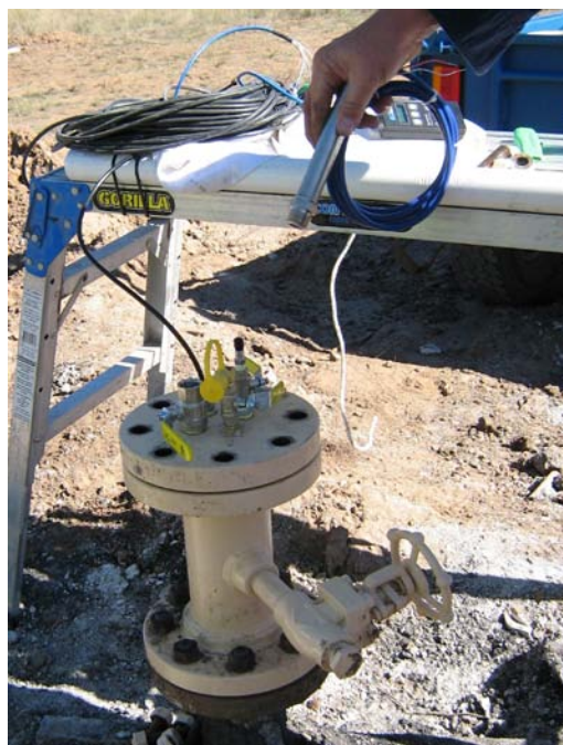
Figure 4. Ground water monitoring station
