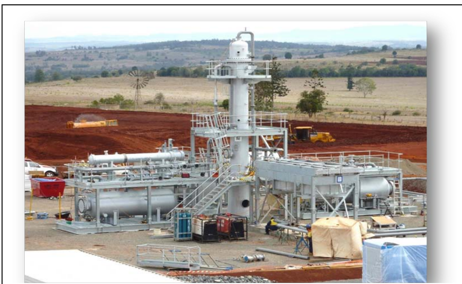
Gas Processing Plant
