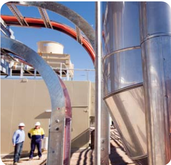
Wilga Park Power Station
