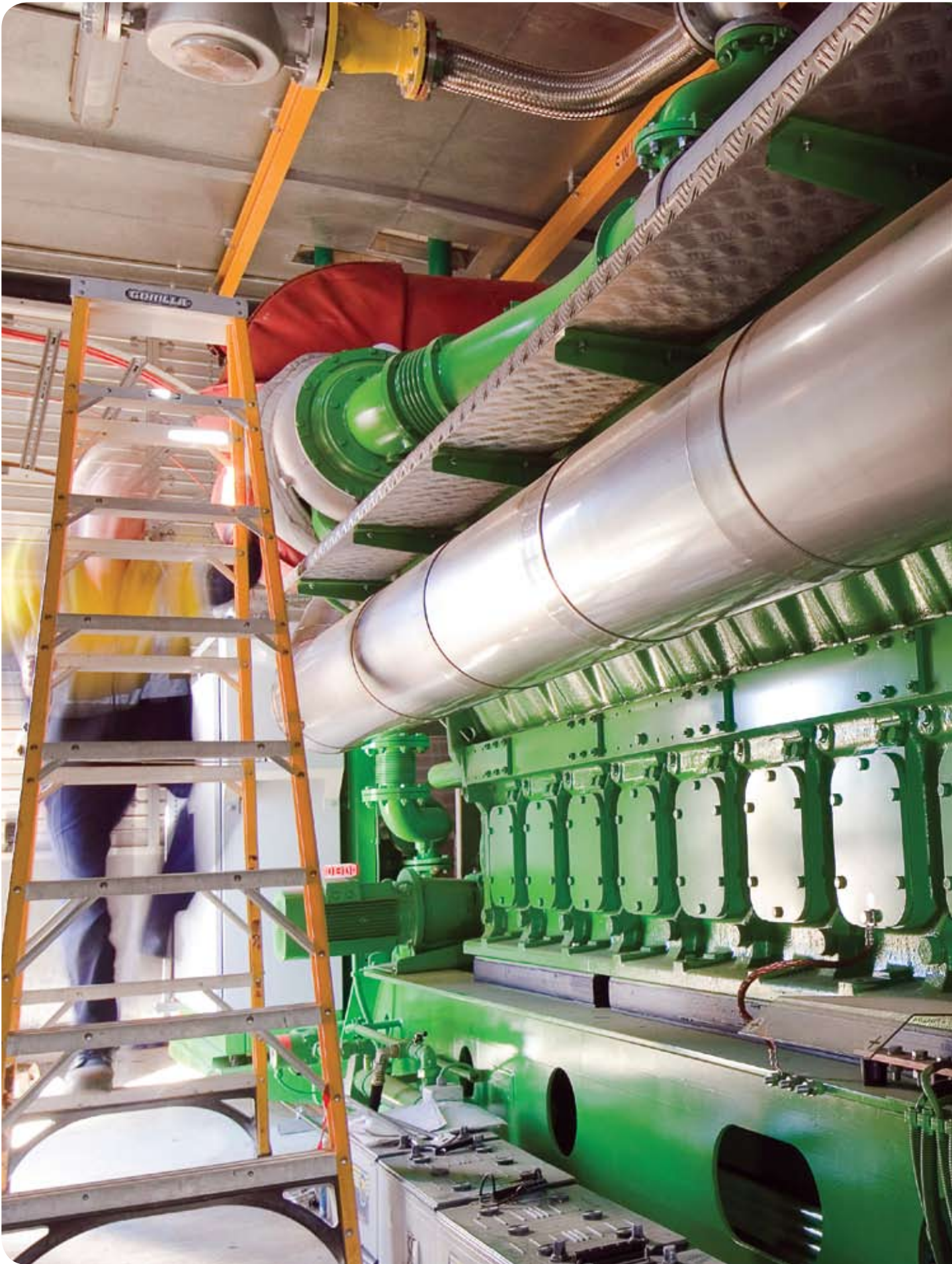
Gas fired generator at Wilga Park Power Station
