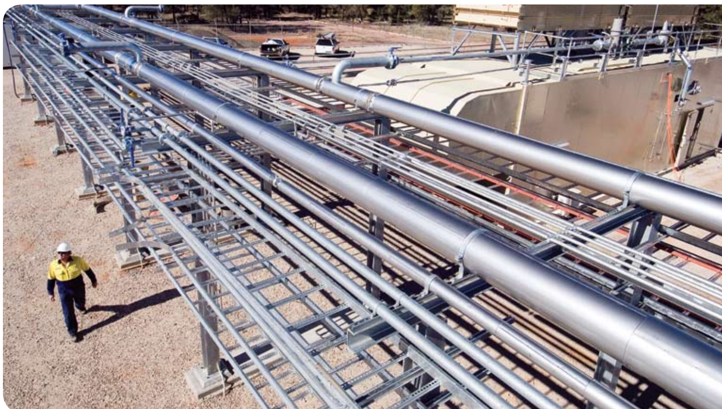
Wilga Park Power Station prepared for future expansion
