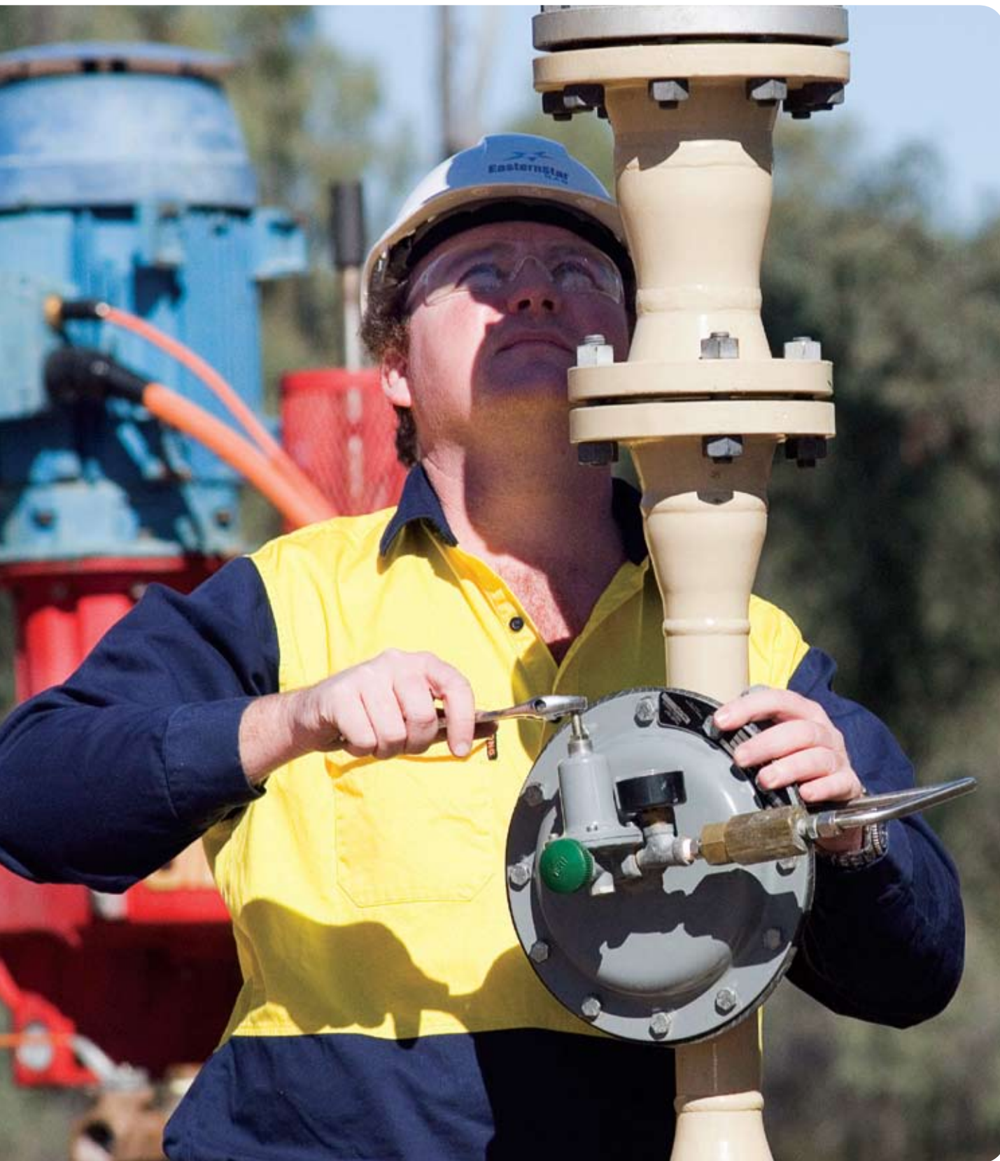
Adjusting separator pressure at Bibblewindi Lateral Pilot
