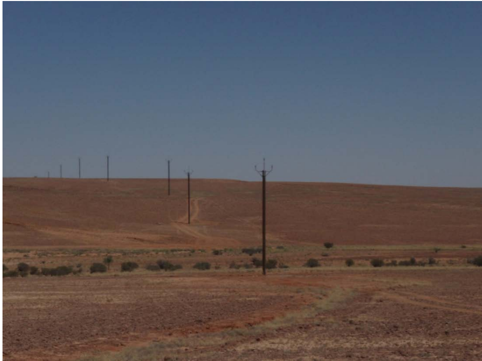
Power poles between the Habanero site and Innamincka township
