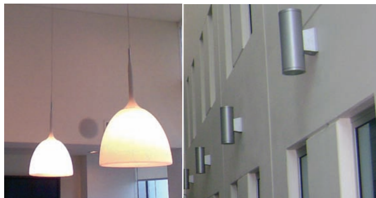
Customised light fittings at Andel Holdings
