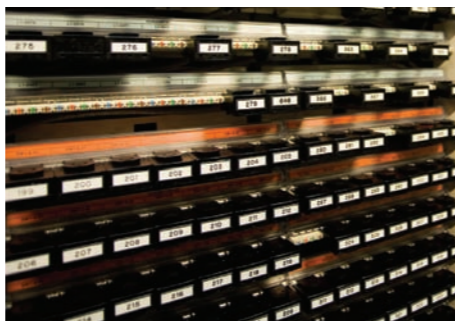
Communications patch panel
