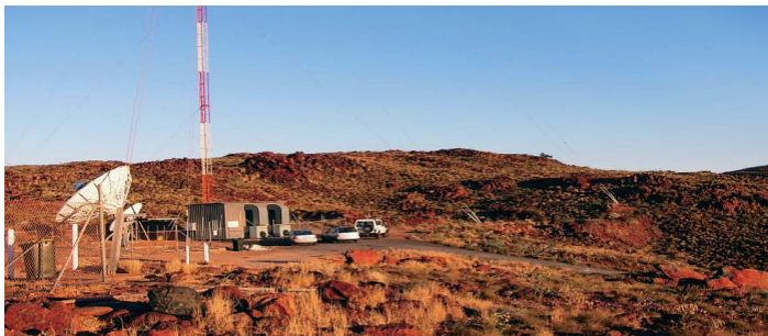
Broadcast Australia is the owner and operator of one of the most extensive terrestrial broadcast transmission networks in the world.
