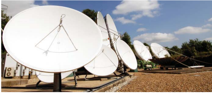
Arqiva owns, manages and operates a global teleport infrastructure including over 100 major uplinks at 10 teleports with on-site co-location and data hosting.
