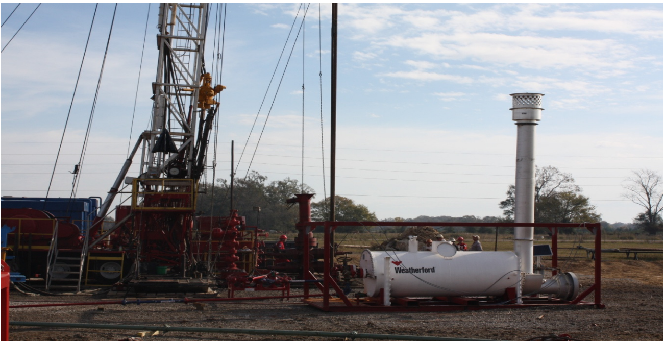
Perforation of the HM Brian No.1 well and associated testing equipment supplied by Weatherford
